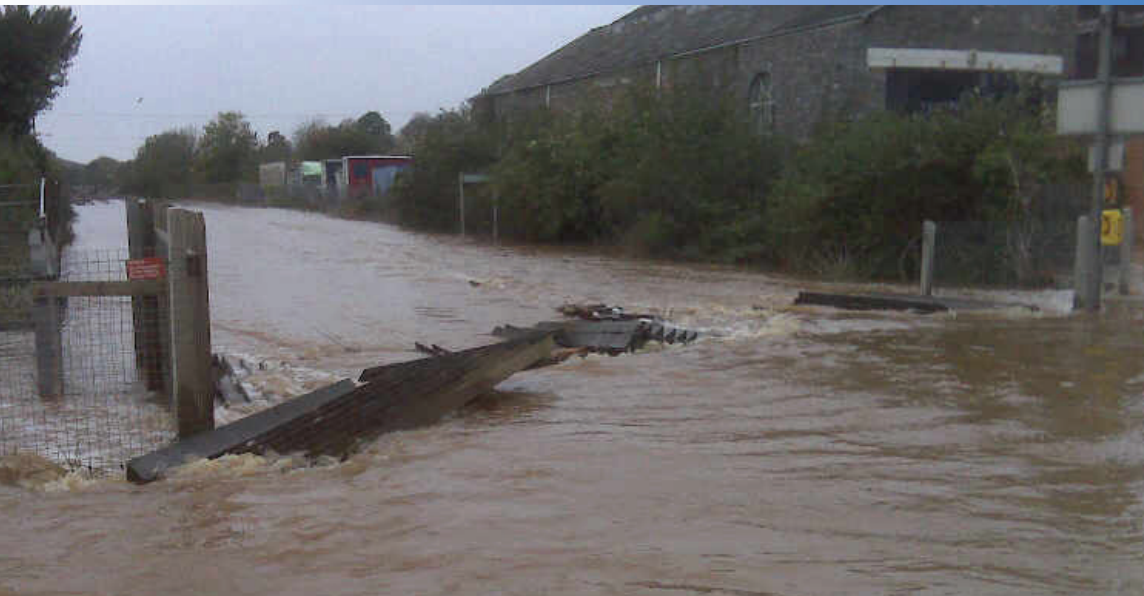
▲ At first glance this image could be said to be a local river in full flow having burst its banks - alas it is actually Network Rail's Great Western mainline between Exeter St. Davids and Tiverton Parkway! The track at this point being around two-feet under water. Network Rail
